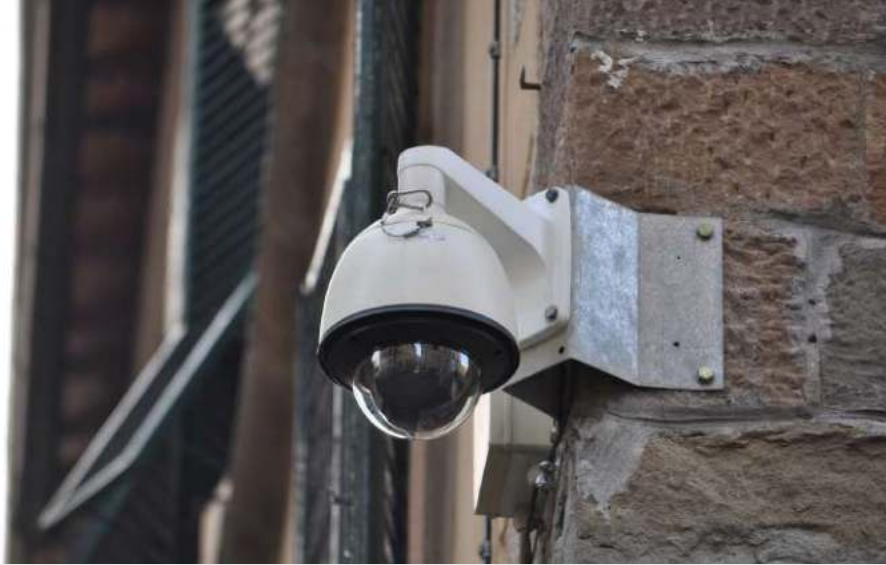
A Closed Circuit Television (CCTV) camera mounted on a wall.
