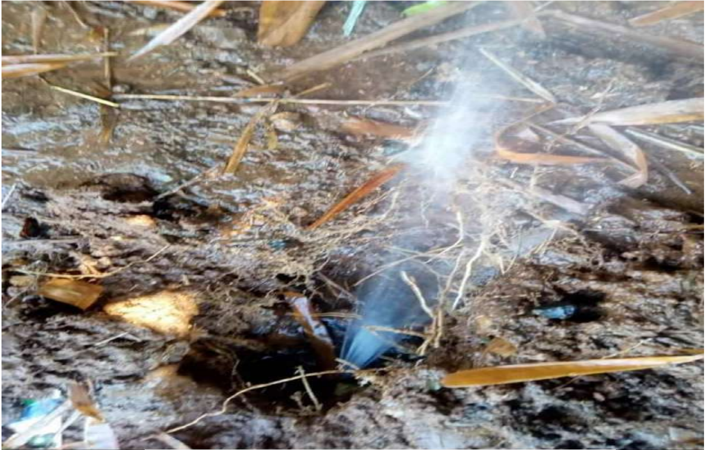
A jet of water splashes out from leaking water pipe / Photo courtesy of MAWASCO
