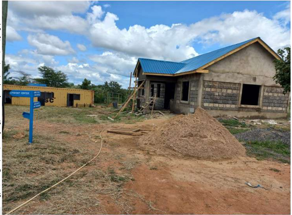
Above and below: Ongoing construction of KEWI Kitui Campus Administration Block and erection of the borehole mast.
