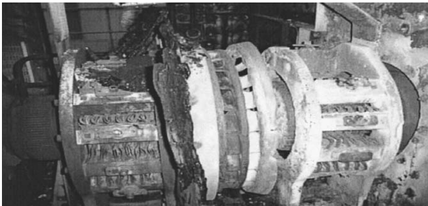
FIGURE 18.3 Collector and brush holder neglect.
