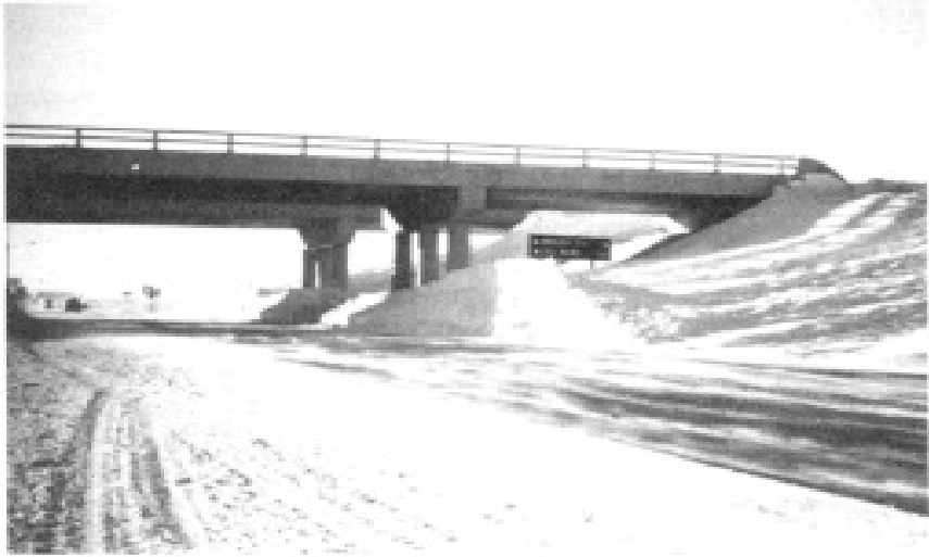
Figure 5.10 Adjacent appurtenances create unwanted snow drifts on the roadway.
